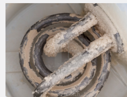
Example of lime-scale deposits from hard water areas.
